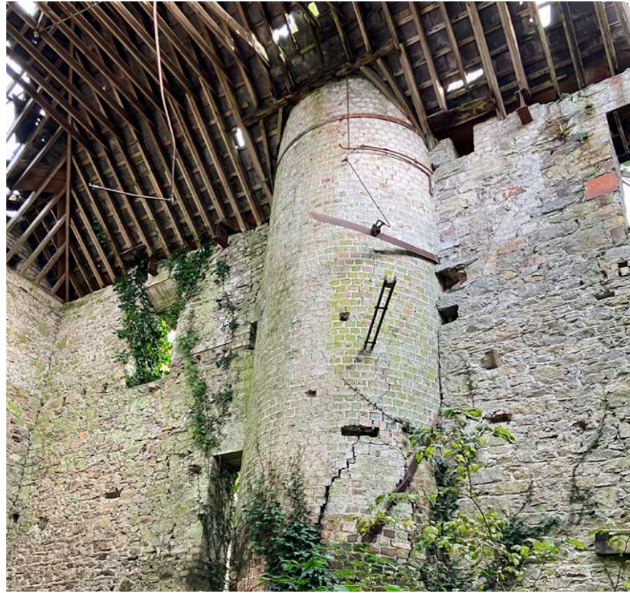
Figure 71 - Kiln/engine house structural damage to cross wall.
