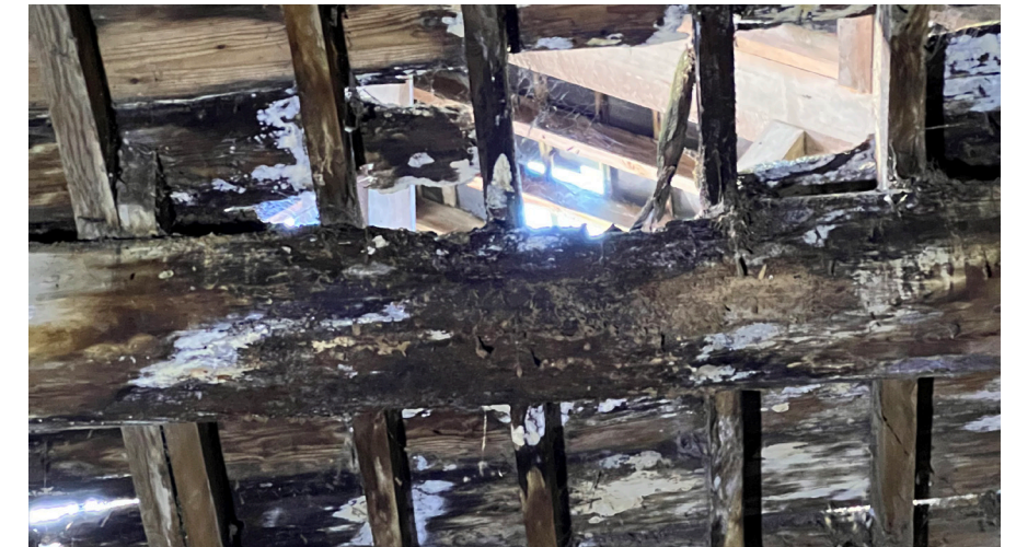
Figure 132 - Malt house - water damage to floors.
