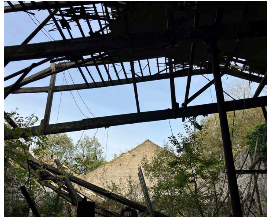
Figure 116 - Long shop - collapsed roof at east end.
