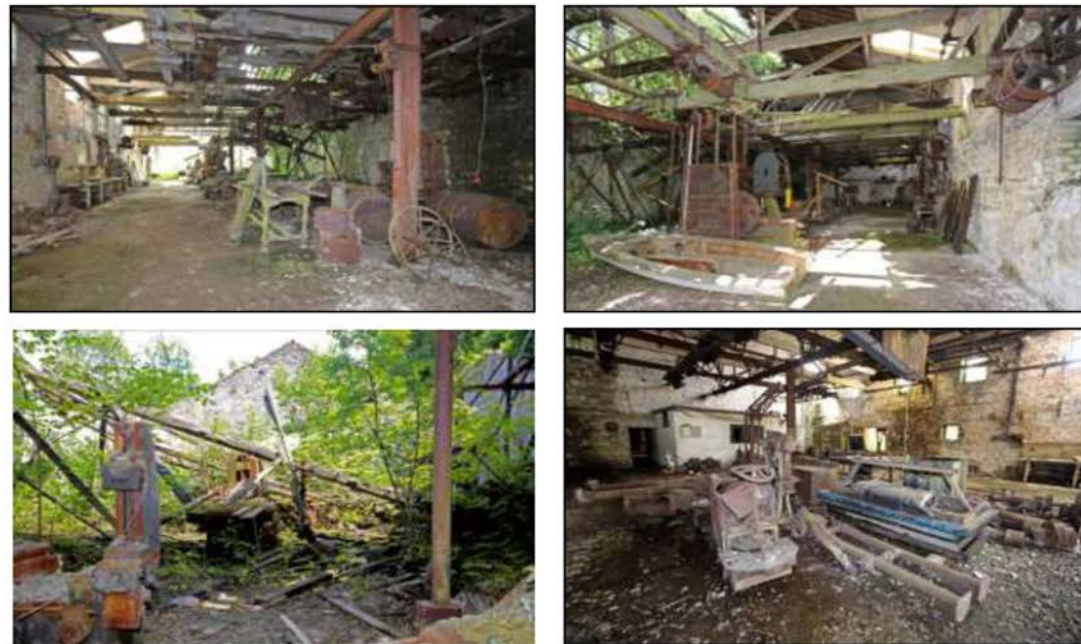
Fig.4 General views of items in Building 2: Top left: Looking E along N side of room. Top right: Looking E along S side of room. Bottom left: Collapsed roof at E end of building. Bottom right: Looking W along N side of room.
