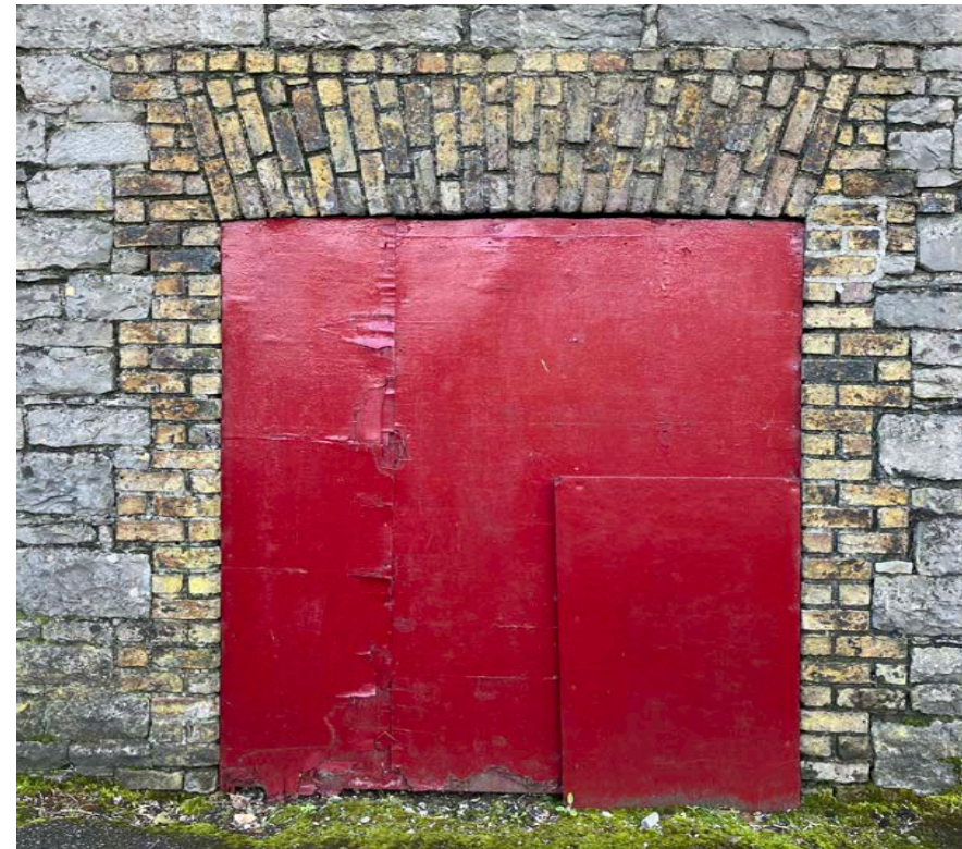
Figure 131 - Warehouse/cooperage blocked external doorway.
