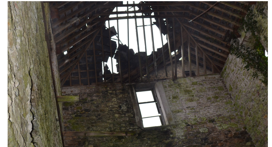
Figure 92 - Kiln/engine house underside of badly damage roof.
