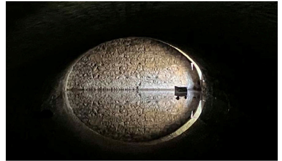
Figure 58 - Bonded warehouse flooded west end.
